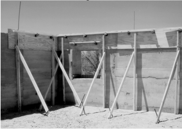
Figure 6. “Flying formwork” for the bond beam was difficult to support and level.
